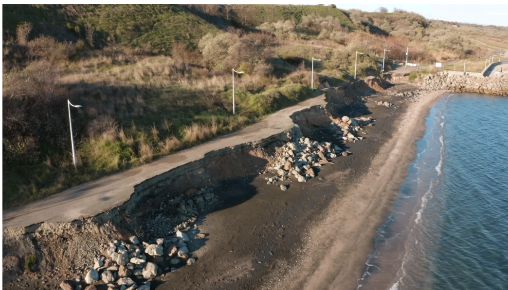
Picture 4: Damaged coastal trail between Burgas' city centre and Sarafovo.
